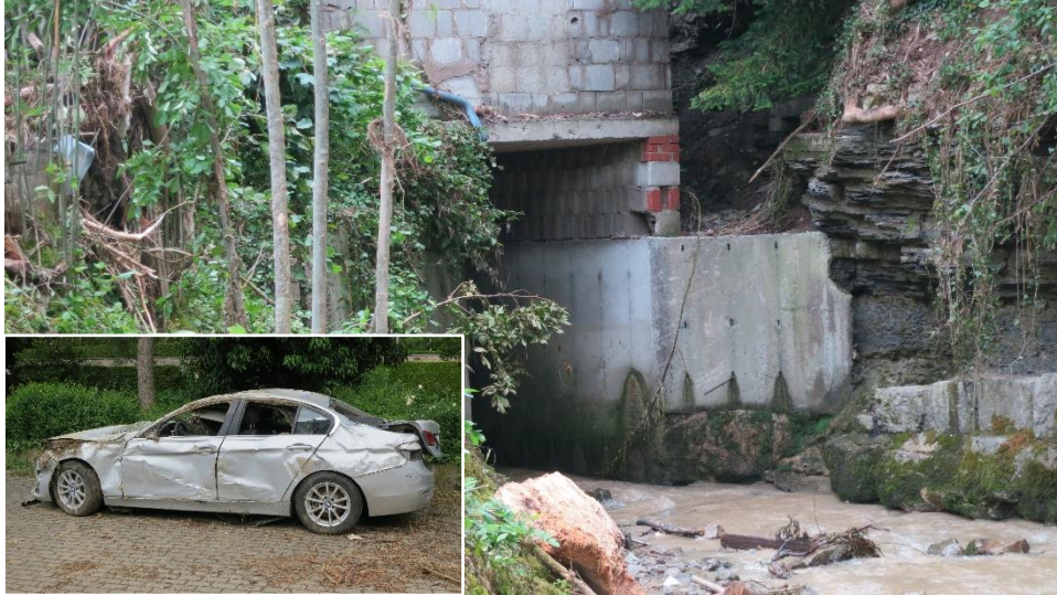
Figure 17: Entry to an underpass of a building, which was blocked by a motor vehicle during the High Water.
