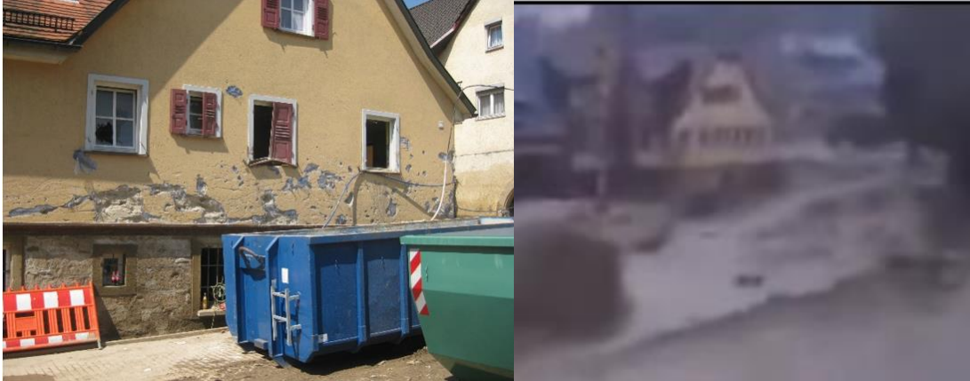
Figure 11: Damage at the Ground Floor (Souterrain/Deep parterre) and First Floor (left); Flow Situation during the Event with Locally Strong Varying Water Levels (right).
