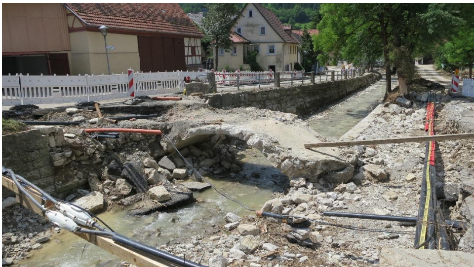
Figure 14: Damage to streets after a flow-around at a bridge in Steinkirchen.
