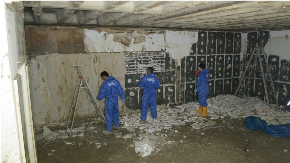
Figure 18: Remediation work at a building in Künzelsau. Because of the moisture damage a dismantling of the basement and ground floors to shell construction status is required in many cases.
