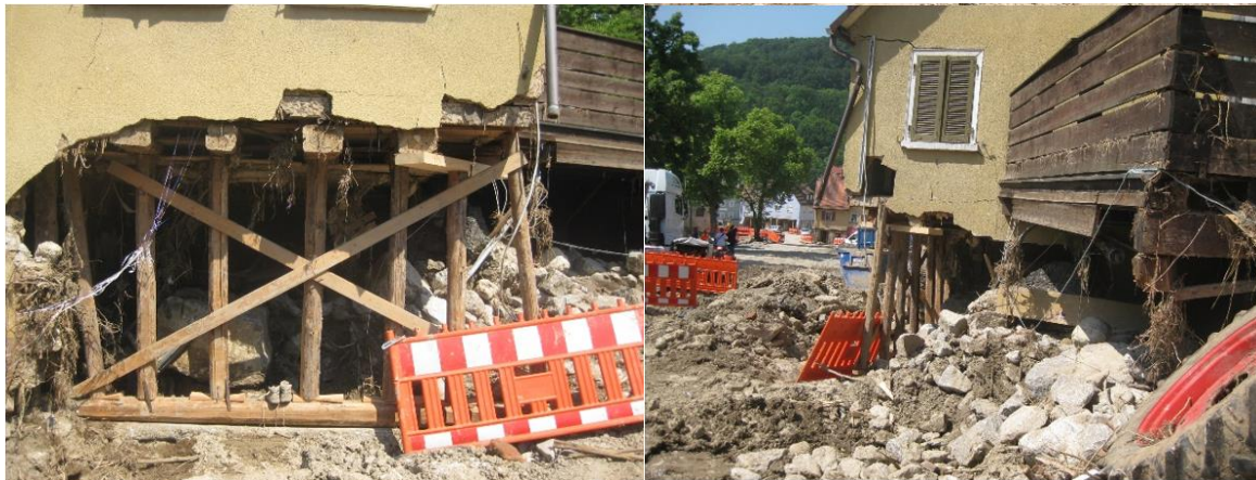
Figure 12: Structural damage to buildings in Braunsbach.
